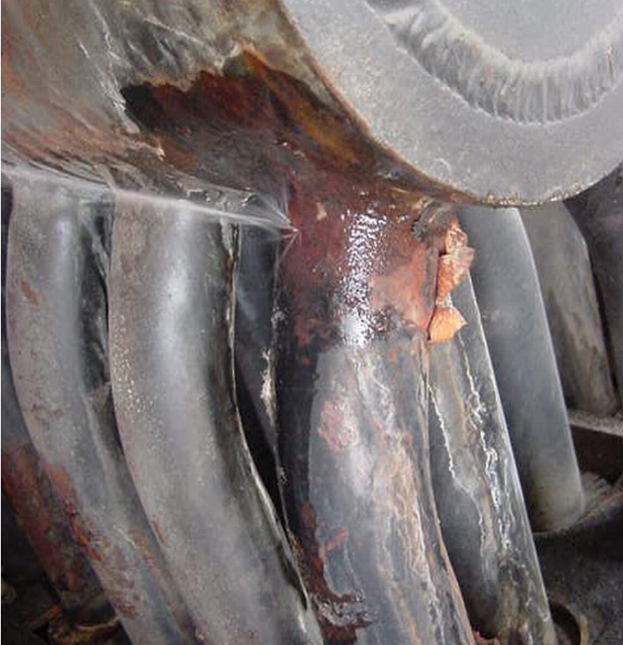
Figure 3-24 Corrosion Fatigue Appearance – Pin Hole Leak
