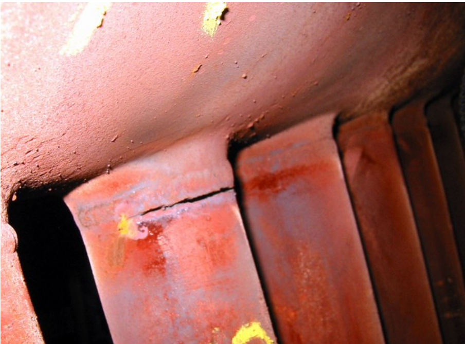
Figure 3-25 Corrosion Fatigue Appearance – Crack
